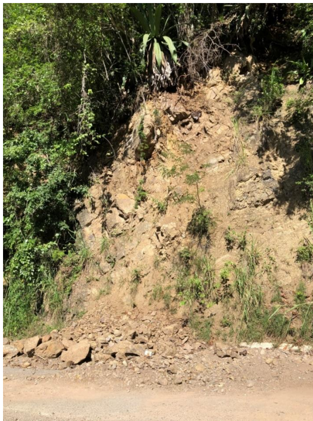
Figure 5-11: Erosion near Irish Town (18.04532N -76.72725W)
